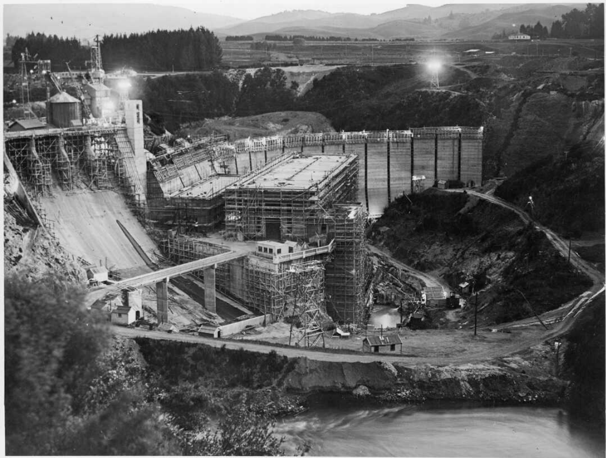
Figure 69: 'Karāpiro Hydroelectric Power Plant Under Construction', January 1946, New Zealand Free Lance , no. 6, vol. 1 (1946). Image: Alexander Turnbull Library, PAColl-7171-00079, CC.BY.4.0.
