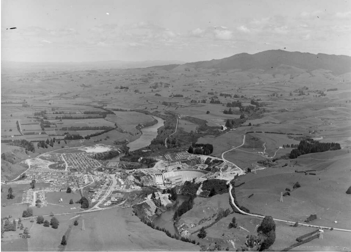
Figure 68: Whites Aviation, 'Construction of the Karāpiro Hydroelectric Power Station, including the Waikato River, Karāpiro, Waikato' with Maungatautari in the background, 20 November 1946. Image: Whites Aviation Collection, Alexander Turnbull Library, WA-04409-G/PA-Group-00080, CC.BY.4.0.
