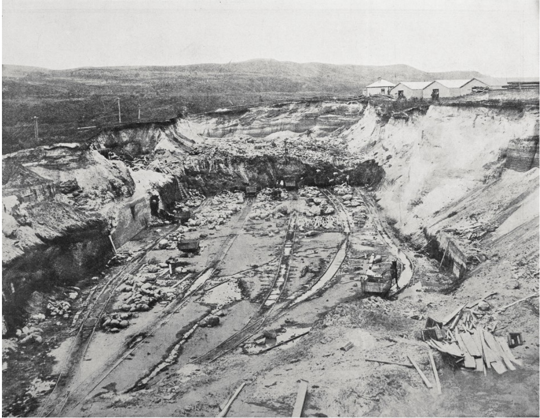
Figure 64: "Practically a New River Bed: Cutting the Race at the Horahora Rapids Electric Power Works, Waikato," Auckland Weekly News (16 February 1911), 7. Image: Auckland Libraries Heritage Collections, AWNS-19110216-7-2, CC.BY.4.0.
