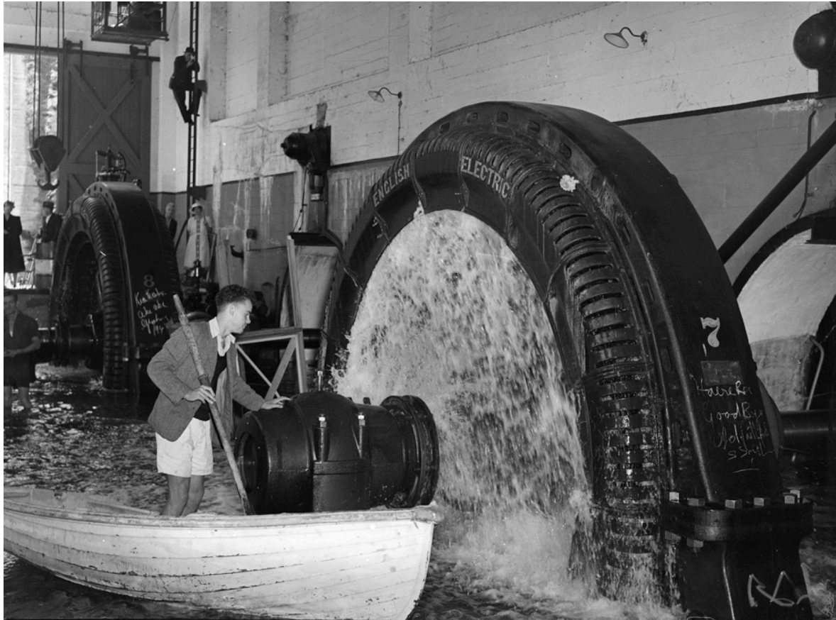
Figure 70: The flooded interior of the Horahora Hydroelectric Powerstation showing the number 7 generator, which would not shut down. Note Kiwa Graham's inscription on the number 8 generator (background). Image: Auckland Libraries Heritage Collections 1370-231-8, CC.BY.4.0.
