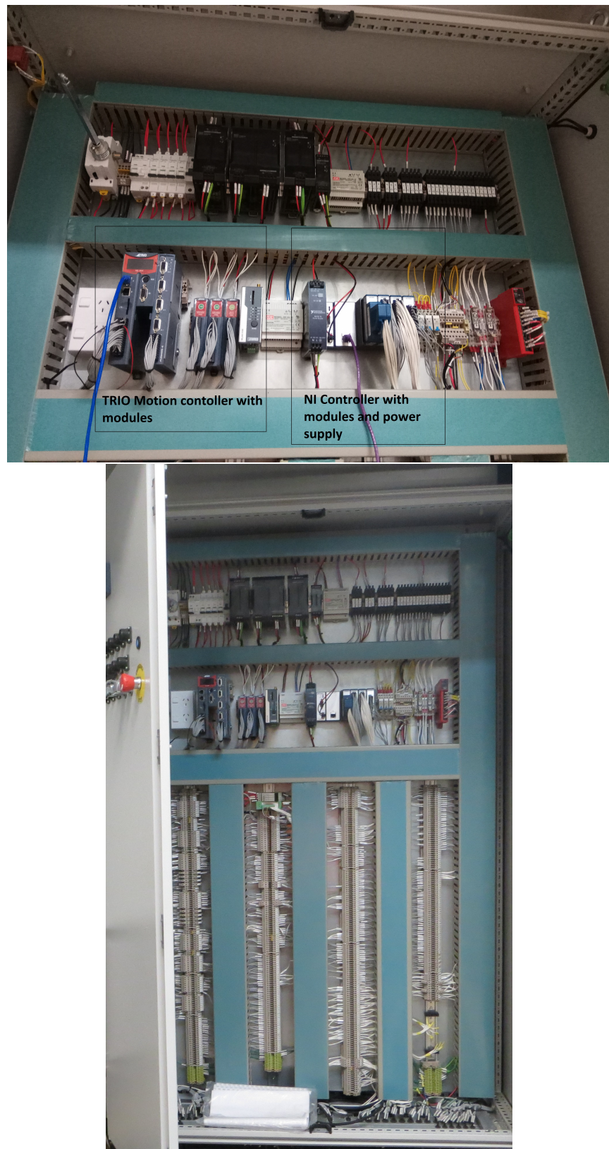
Figure 4.5: Low voltage cabinet of the ss-CAES prototype.
