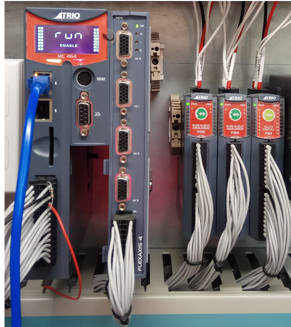
Figure 4.6: TRIO Motion controller MC464 with two analog modules P326 and a digital module P319 in the low voltage cabinet of the ss-CAES prototype.
