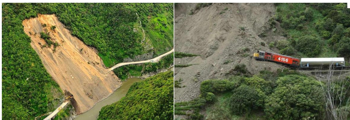
Figure 1.1: Landsliding in the Manawatu Gorge, New Zealand. Photo courtesy of NZTA (left) and Warwick Smith (right).
