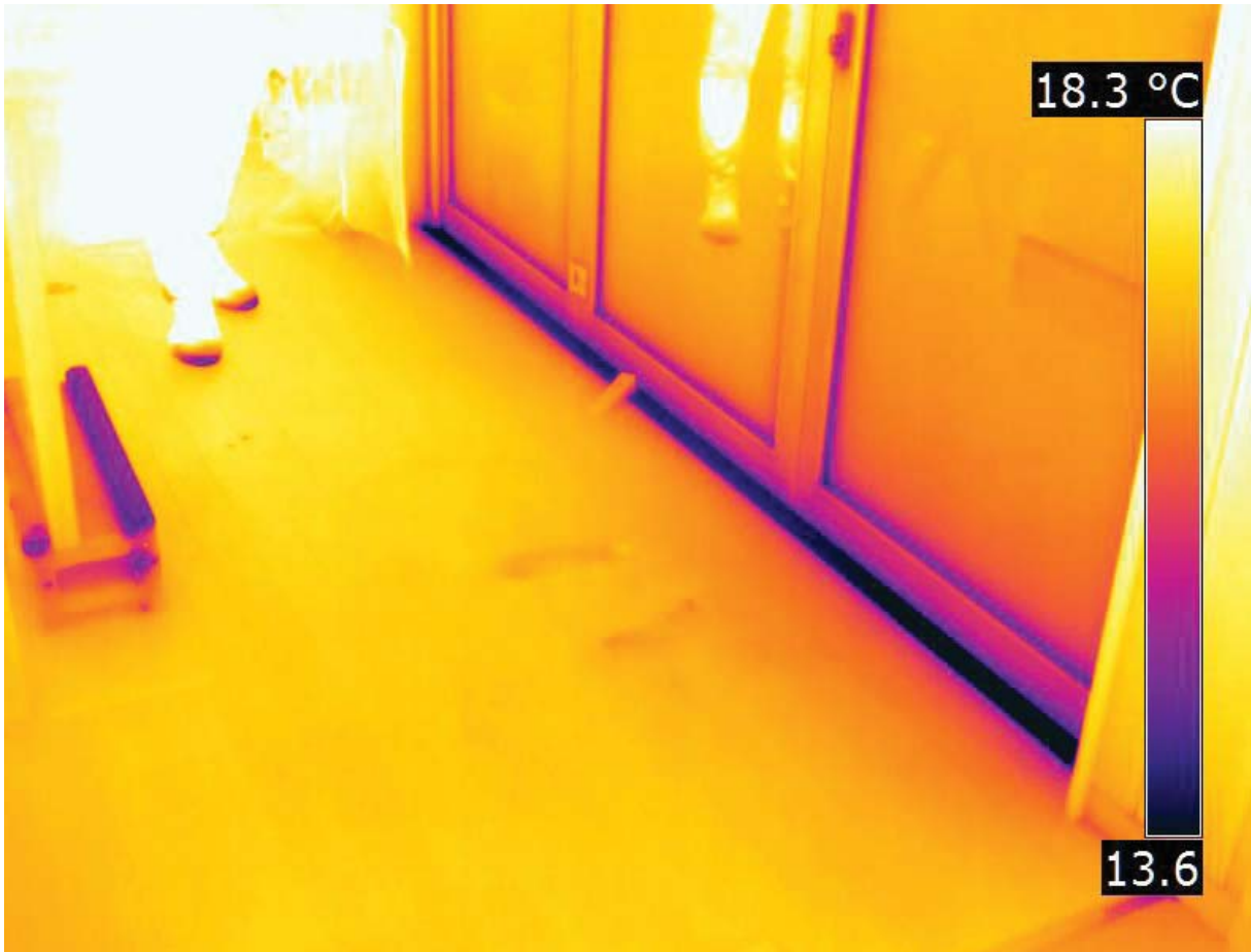
Figure 88: Faulty seal at the base of the bifold doors (Source: Image courtesy of BRANZ)
