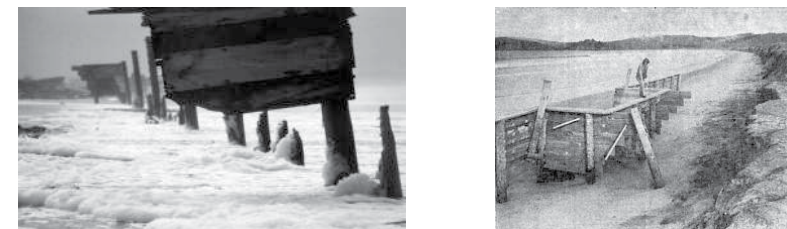
Figures 35 & 36. Erosion and storm damage to the timber seawall at Omaha
