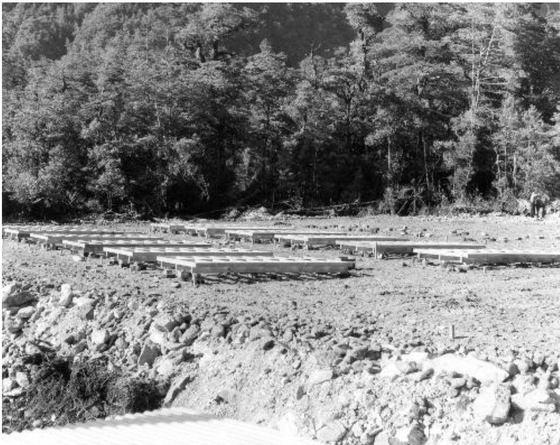
E5: Above ground foundations at West Arm (Photo by Ministry of Works and Development, courtesy of Meridian Energy)
