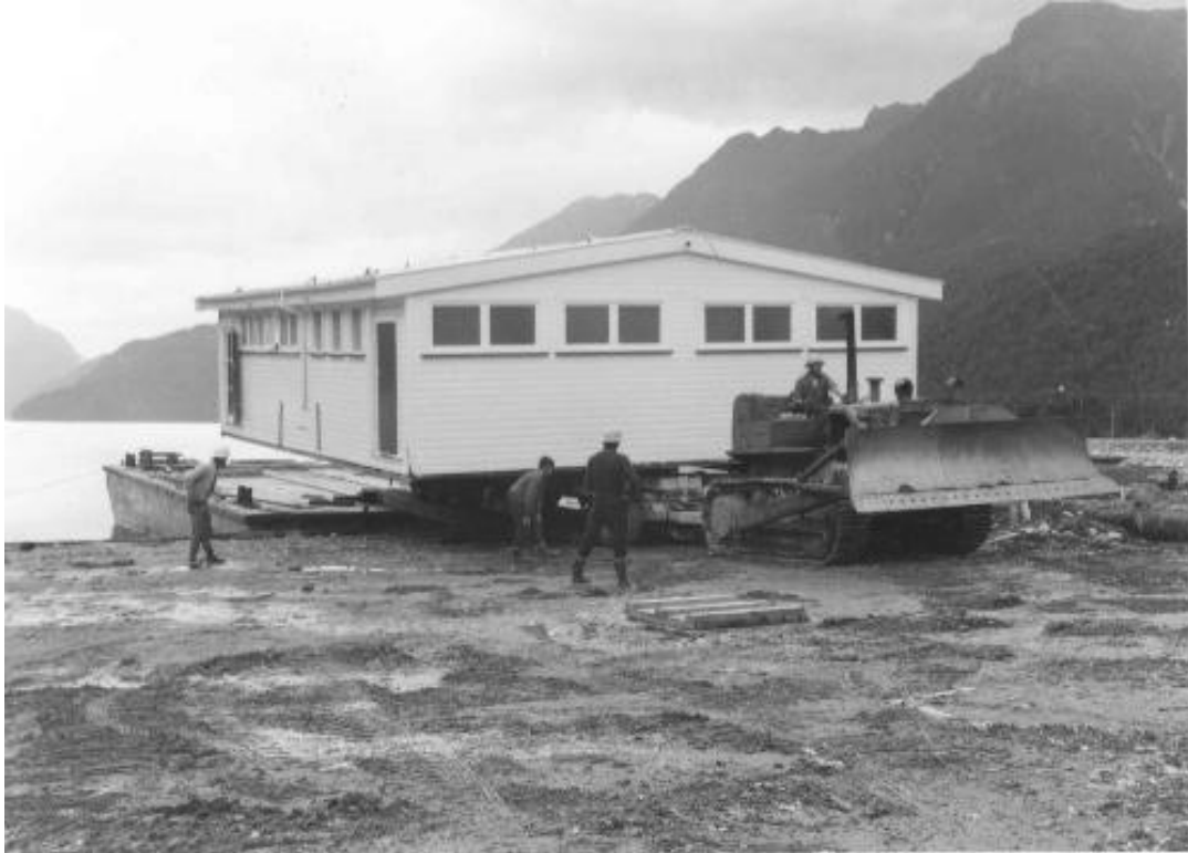
E8: Ablutions block being barged into West Arm. (Photo by Ministry of Works and Development, courtesy of Meridian Energy)
