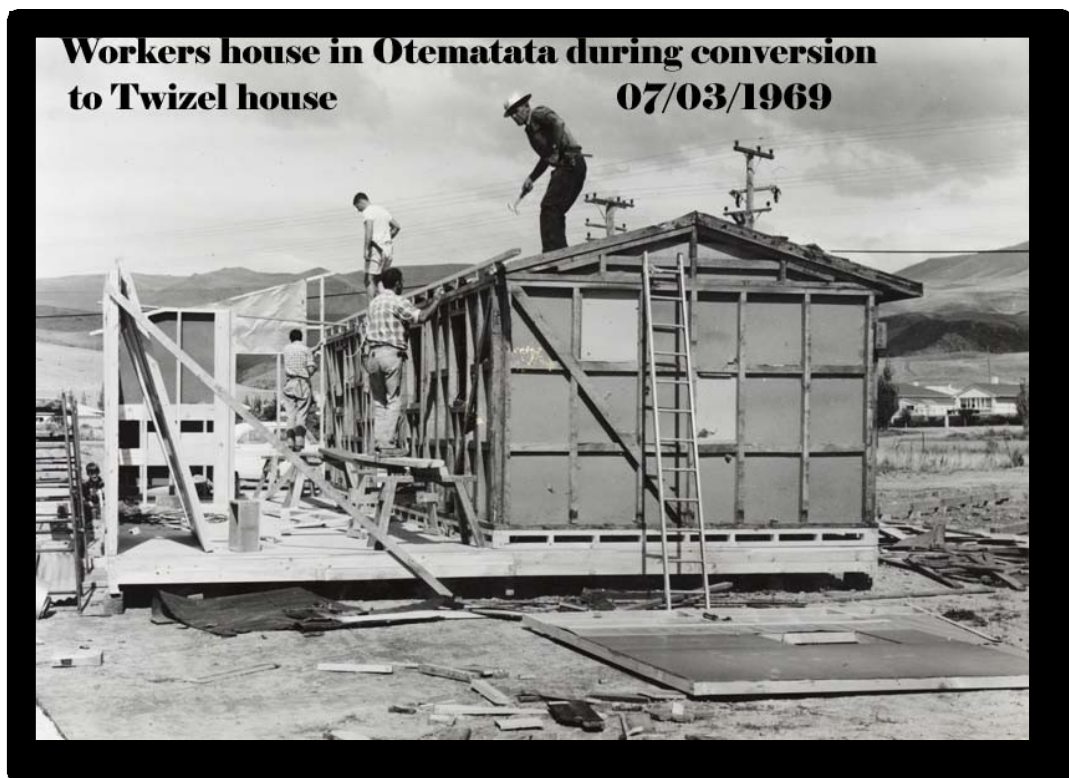
Figure 55: Workers house at Otematata during conversion to Twizel house, 1969 (Photo courtesy of Southern Alps Photos and Gifts)
