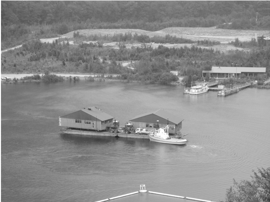
H8: 2MTT hostel sections being barged out of West Arm (Photo courtesy of Meridian Energy)
