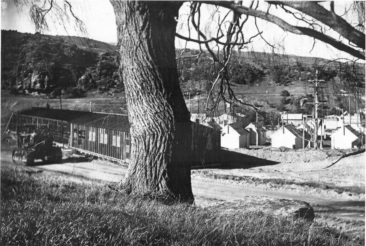
C3: The new block of administration offices being erected in the Roxburgh Hydro Camp. Some of the hutments are also visible.
