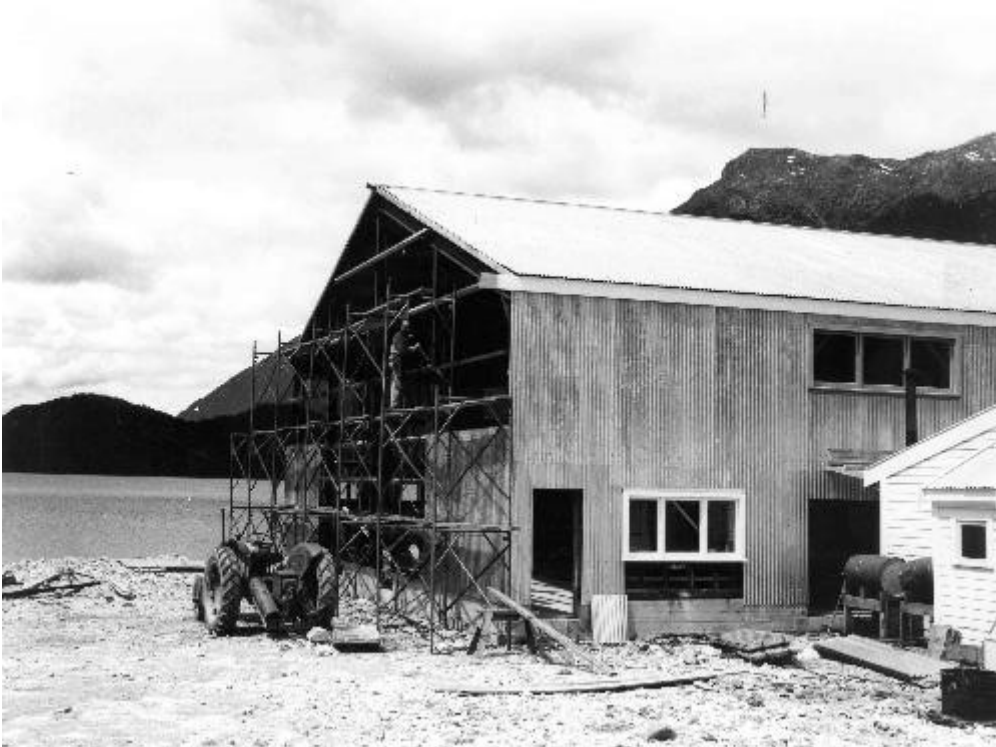
E20: 1MTT staff hostel at Deep Cove under construction (Photo by Ministry of Works and Development, courtesy of Meridian Energy)
