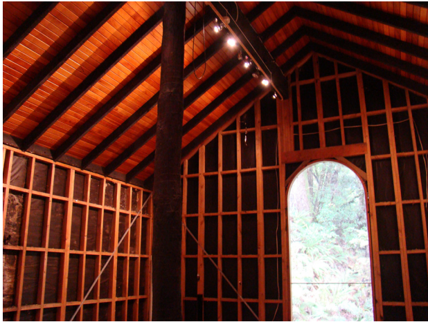
Figure 25. Aniwaniwa Visitors Centre. 'The Maori Hall' With wall lining removed. Image by Author, 2010.
