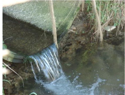
Figure 7.14: "That's the drain pipe...and it looked a bit dodgy" Photographer: Bob, (14, female)
