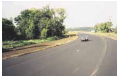
Top Photo: Construction of geofoam road embankment Bottom Photo: New 200' road section completed in 8 working days
