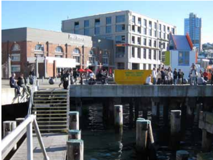
Wharf by Te Papa This part of the wharf has been cut into exposing piles and sea beneath
