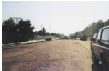
Top Photo: Geofoam blocks being installed in the area of failure Bottom Photo: Compacted base course ready for asphalt application
