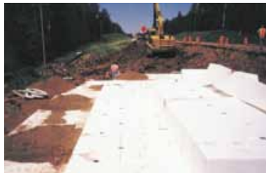
County Highway A Bayfield, Wisconsin For over 20 years, County Highway A had a history of slope failures, and conventional remedies had failed to correct the problem. Geofoam enabled engineers to reduce the landslide driving force without lowering the grade at the head of the slide.
