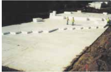
County Highway 12 Elk River, Minnesota Constructed over peat deposits 22'-28' deep, County Highway 12 experienced severe settlement even after previous attempts to correct the problem were made. With minimal excavation, a geofoam road embankment was constructed to reduce the overburden on the underlying poor soils.
