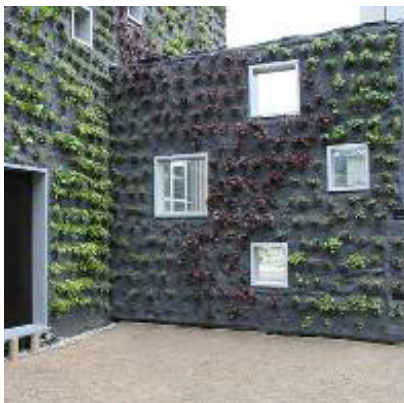
Figure 54: Image of the black box envelope and section through the green wall
