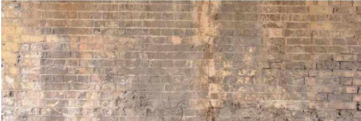
Figure 33: Brick wall damaged by water
